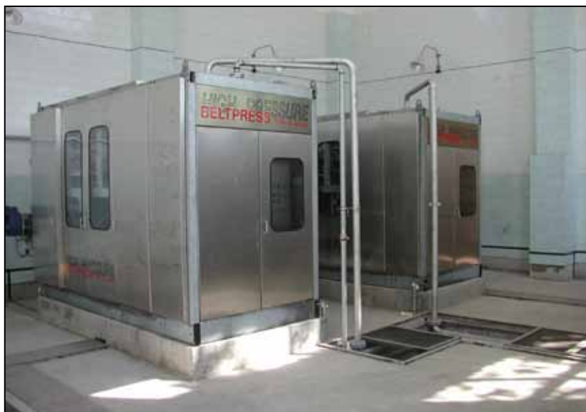
2 x KD 10-1500 - Brest WWTP
